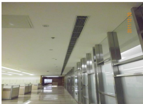
Fig7 Independent temperature and humidity control air conditioning system
