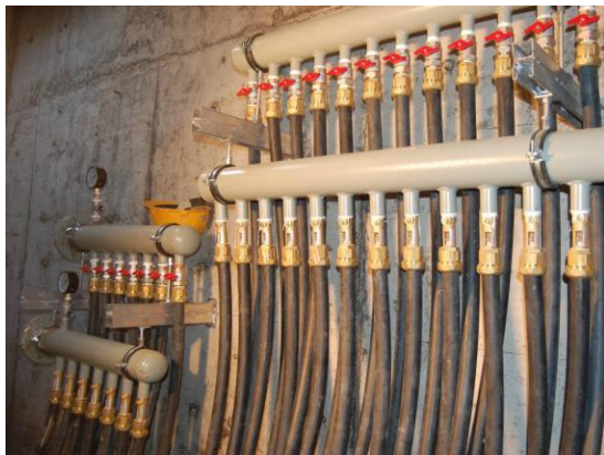
Fig5 Ground-source heat pump system-1
