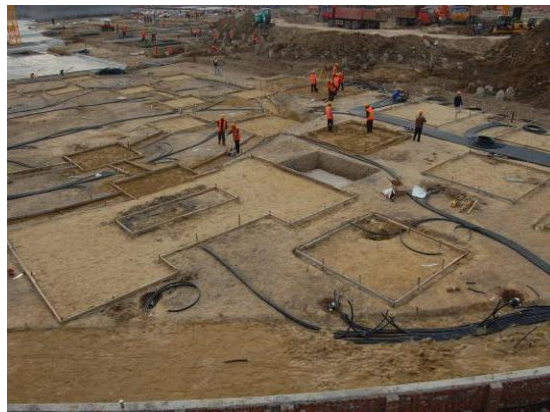
Fig6 Ground-source heat pump system-2
